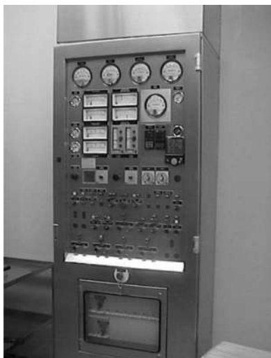
Figure 25 Pneumatic control panel. (Courtesy of the Glatt Group.)
